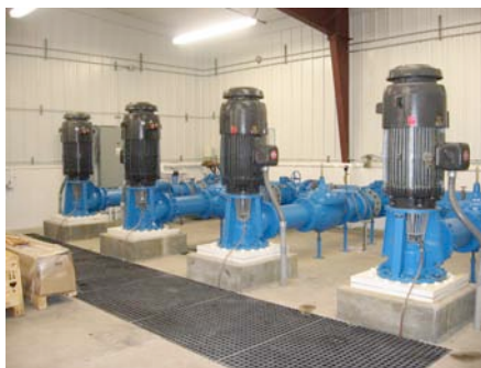
High Service Pumps
