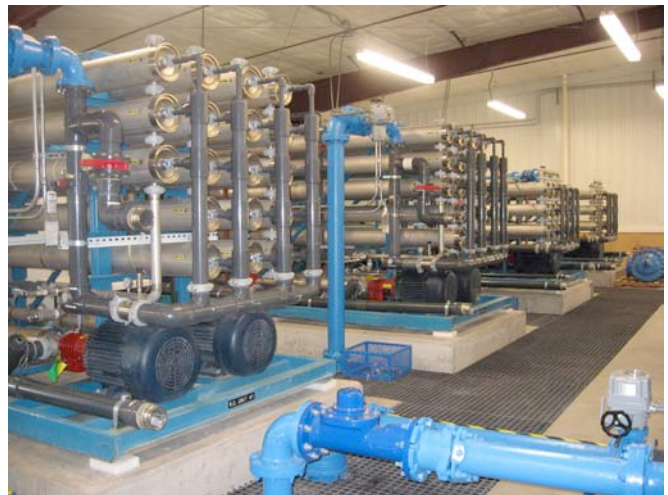
New Torrington WTP Showing Four RO skids
