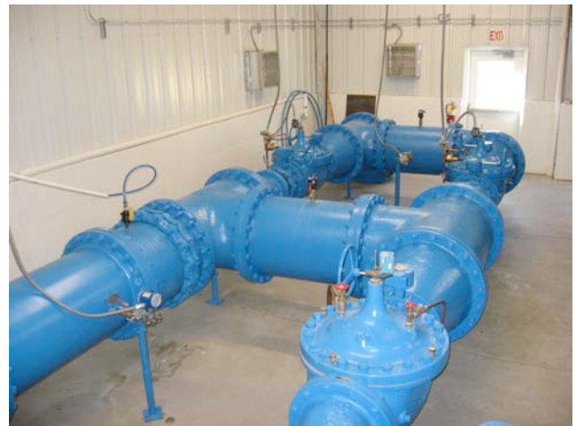
Blending Pipe Gallery Showing Valve
