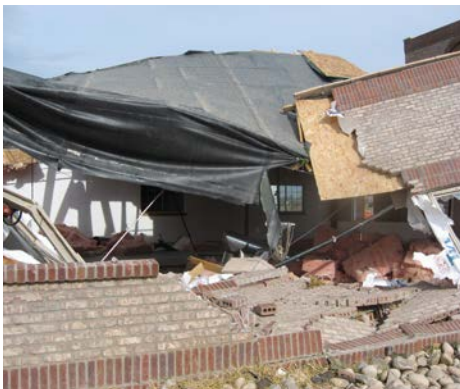
Storm Damage in Town
